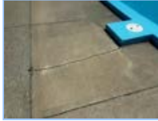
Pool Decking Cracks
