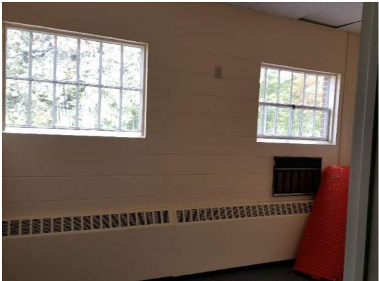
Abandoned Fin Tube Radiation and Thru-Wall Air Conditioner on Lower Floor
