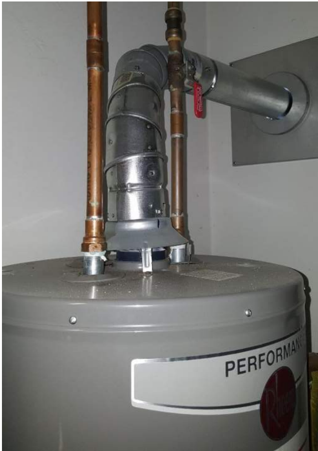
Domestic Hot Water Heater Flue Vent
