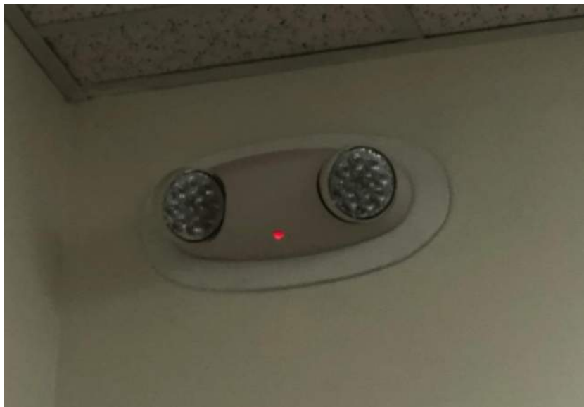
Newer Emergency Fixture
