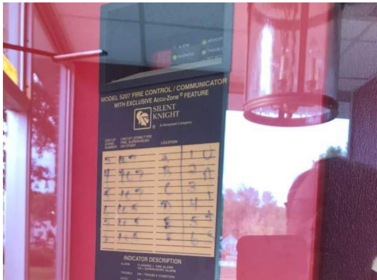
Fire Alarm Panel
