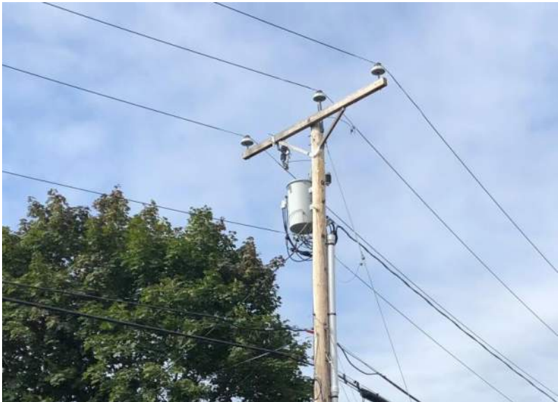
Serving Utility Pole With Three Phase
