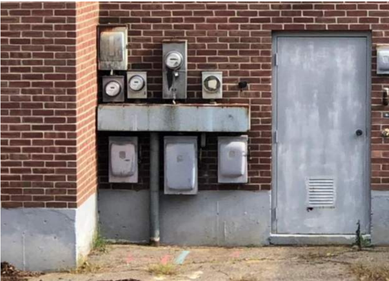
Building Electrical Service/Meters
