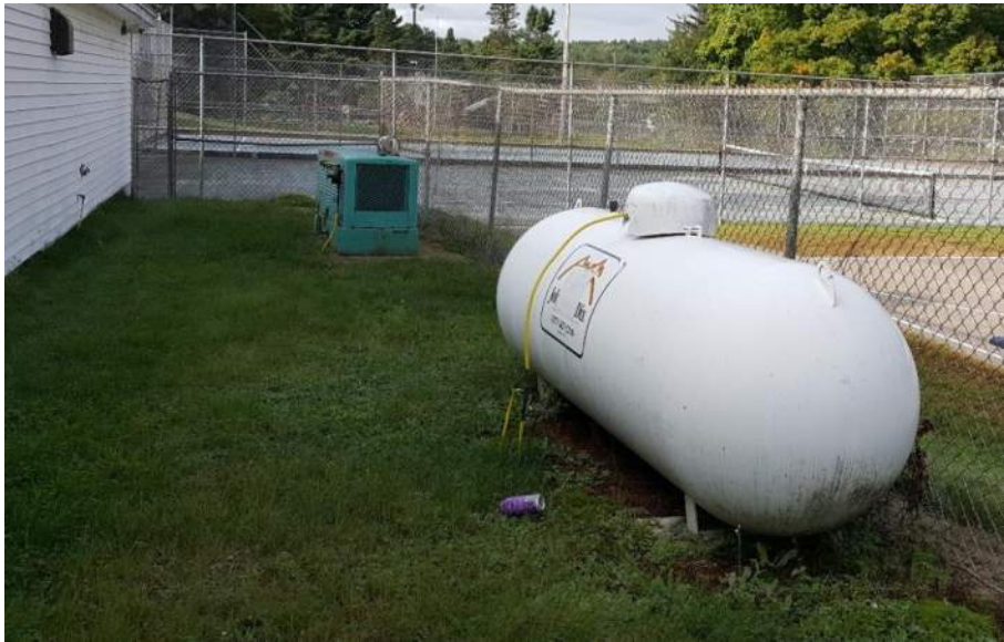
LP Gas Tank and Generator
