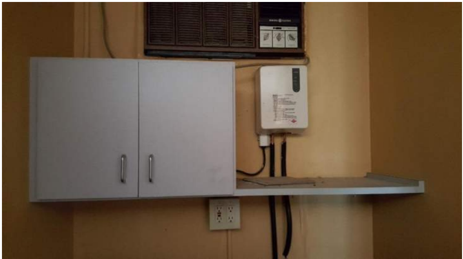
Existing Upstairs Point of Use Water Heater
