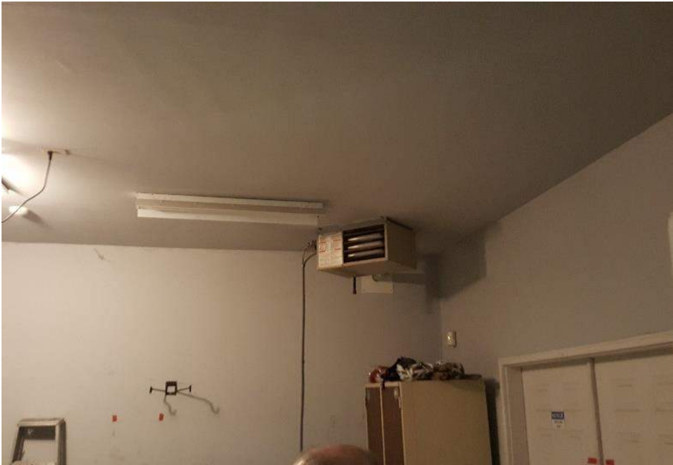
Sally Port Unit Heater
