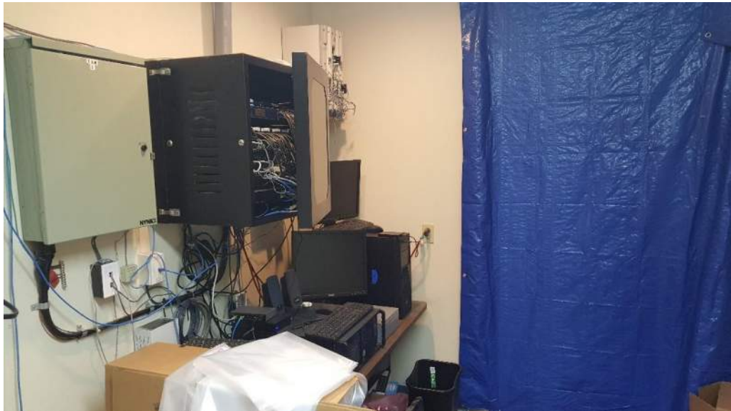
Server and Data Room
