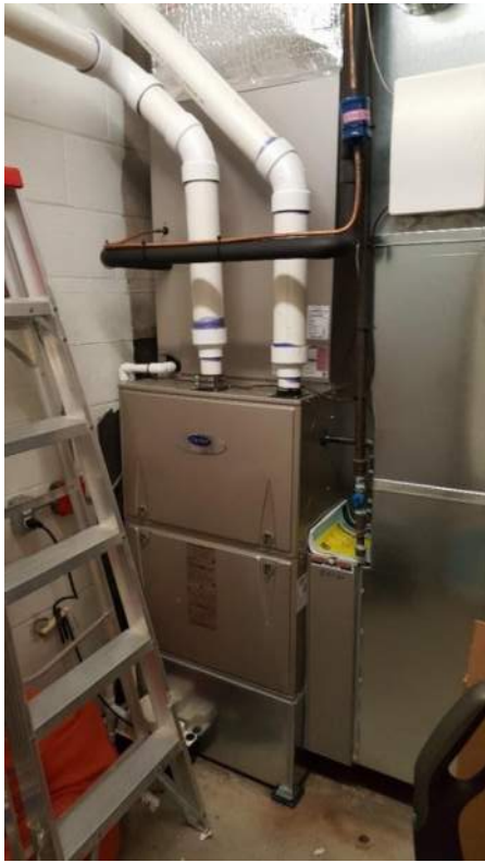
Existing Gas Fired Furnace with DX cooling
