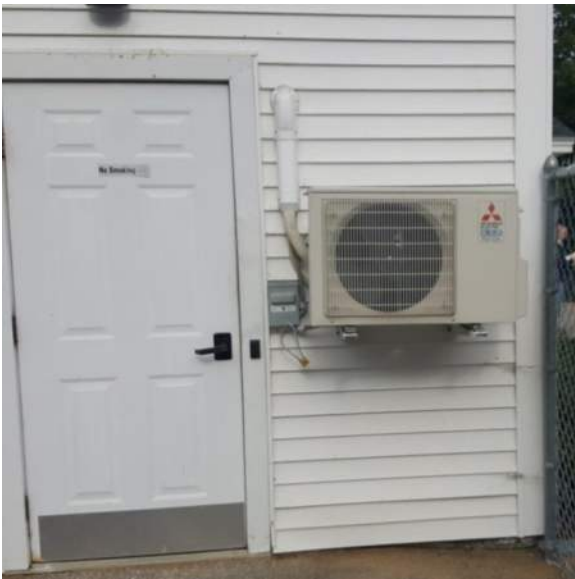
Dispatch Room Outdoor Heat Pump
