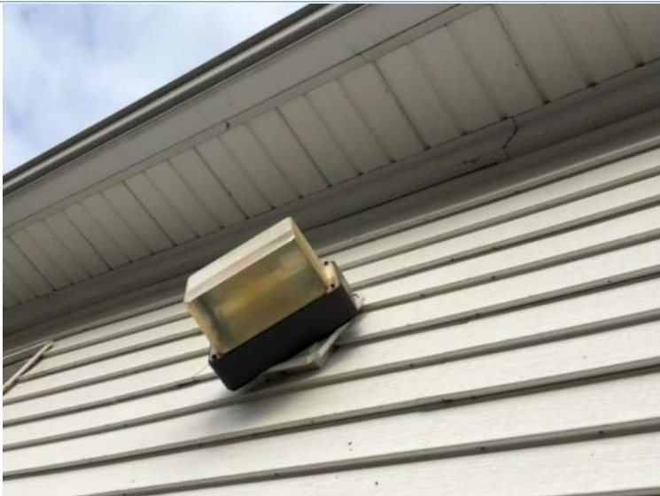
Exterior Metal Halide Fixture
