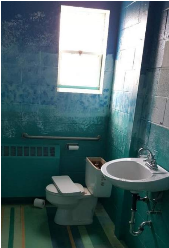
Lower Level Bathroom with Water in Toilet
