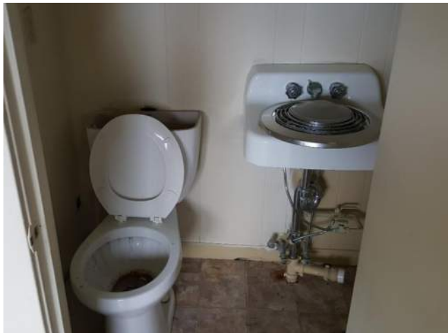
Lower Level Bathroom with Water in Toilet
