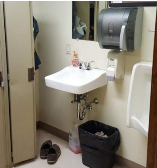
Locker Room Urinal and Lavatory
