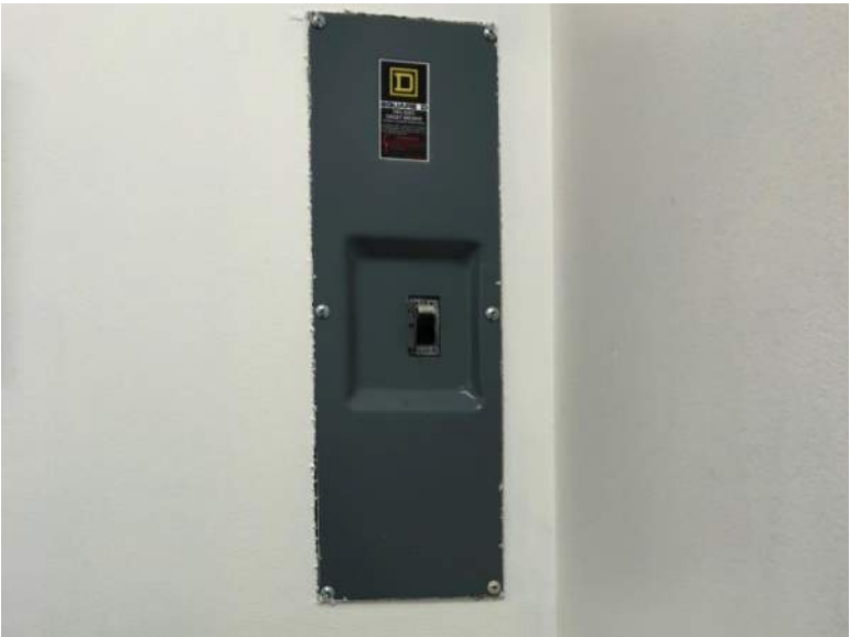
Main Service Disconnect
