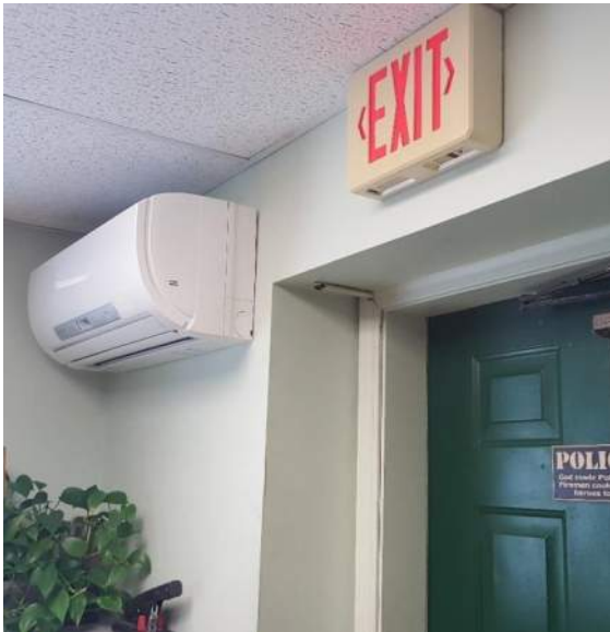
Dispatch Room Indoor Evaporator
