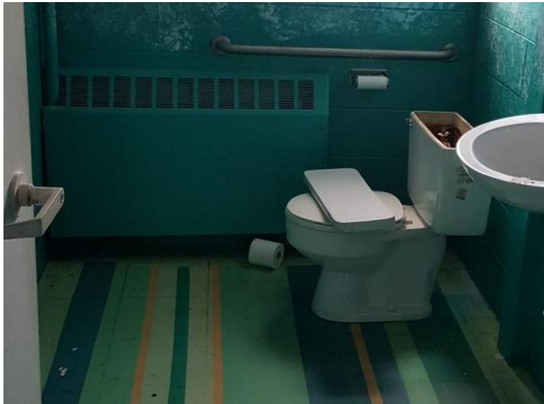
Abandoned Convectors in Bathrooms
