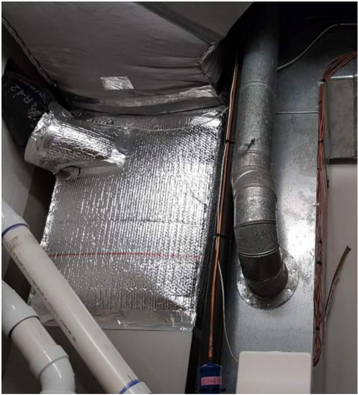
Existing Outdoor Air Duct from Roof
