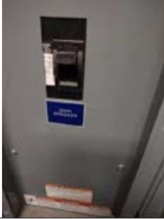
Panelboard for kitchen.
