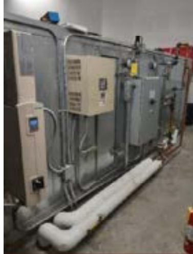
Damper control wiring.
