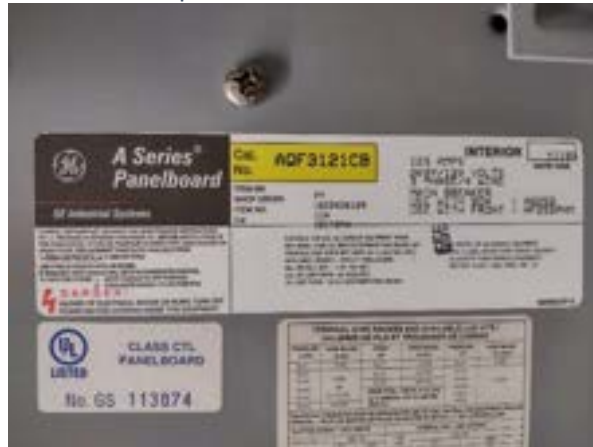
Hallway lighting subpanels - typical.
