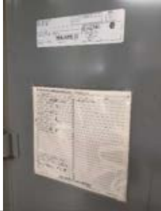
Older main breaker.
