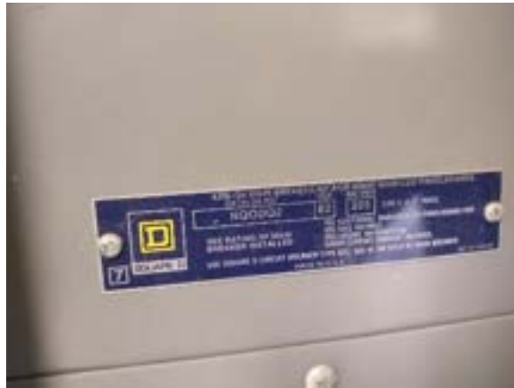
Main breaker showing signs of age.
