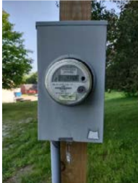
Service Main Panelboard.
