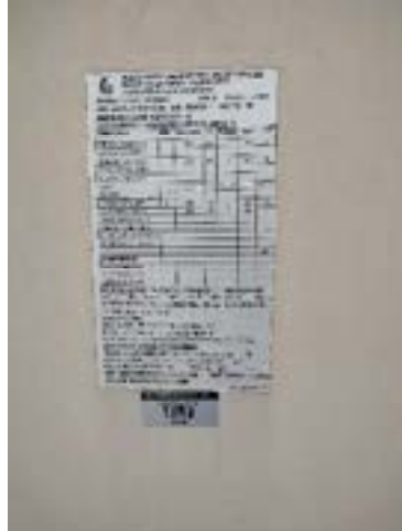
RTU on roof
