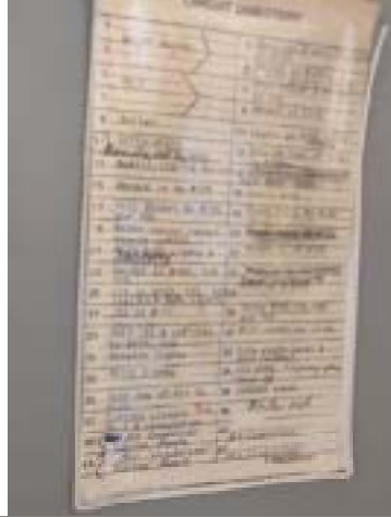
Older disconnect switch.
