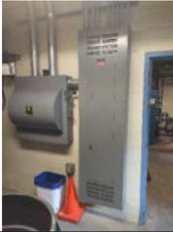
Old main circuit breaker.
