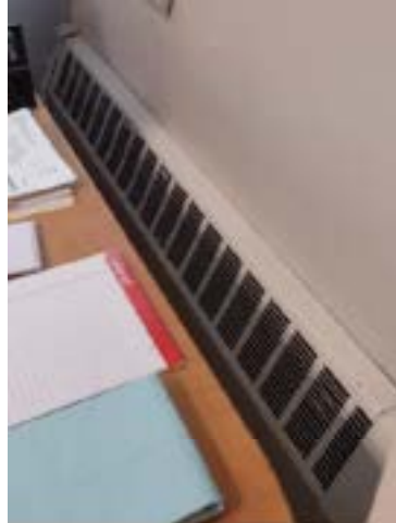
AHU room equipment
