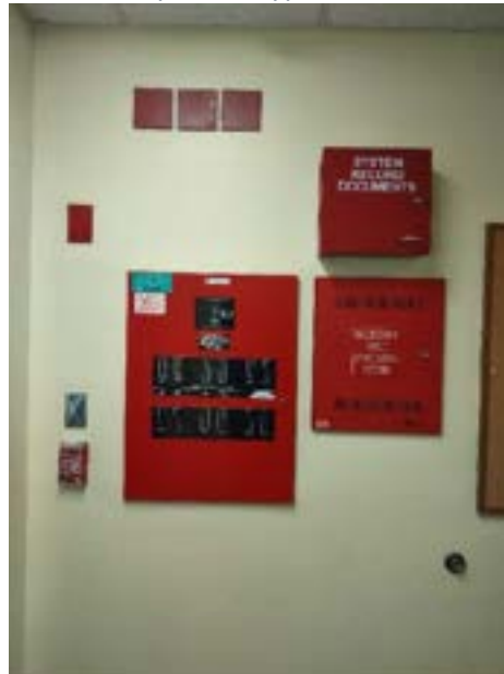
FACP – sub panel – typical
