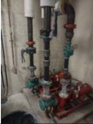
New auto control valves – Very good condition
