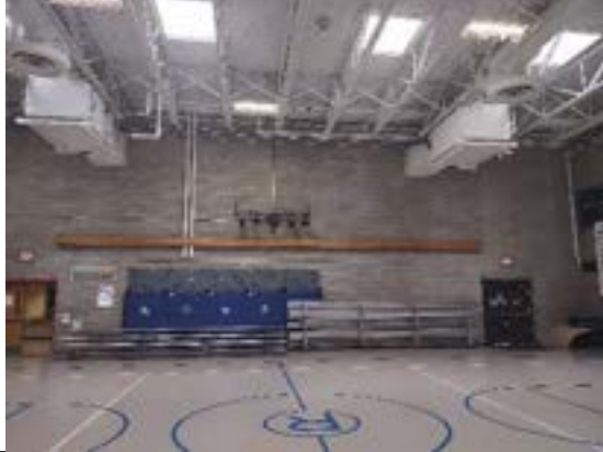
Piping connection to AHU.
