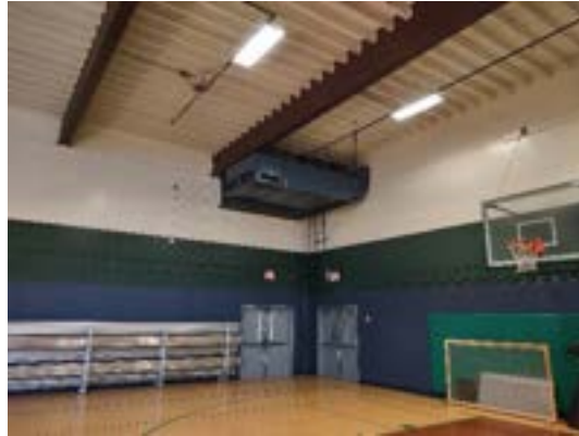
Terminal unit in classroom – typical.
