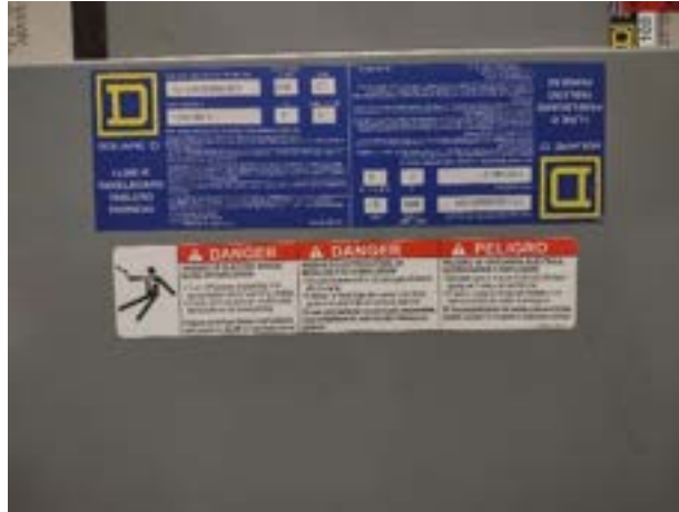
Older panelboard with fire emergency circuit.
