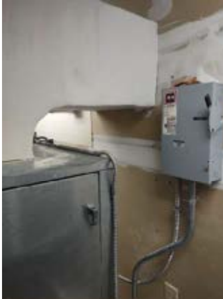
AHU disconnect switch.
