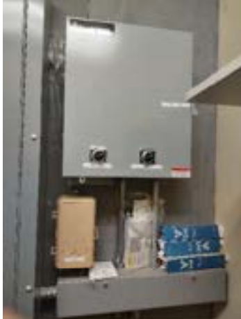
Panel for lighting and outlets – typical.
