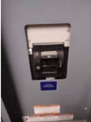
Panelboard for boiler room.
