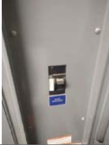
Panelboard shows signs of age.
