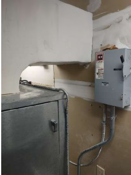
AHU disconnect switch.
