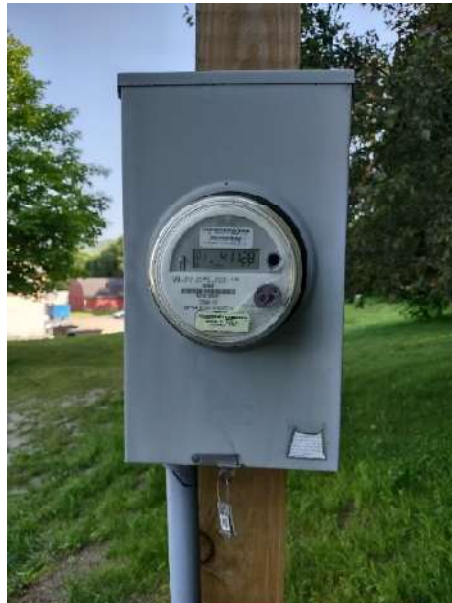
Service Main Panelboard.
