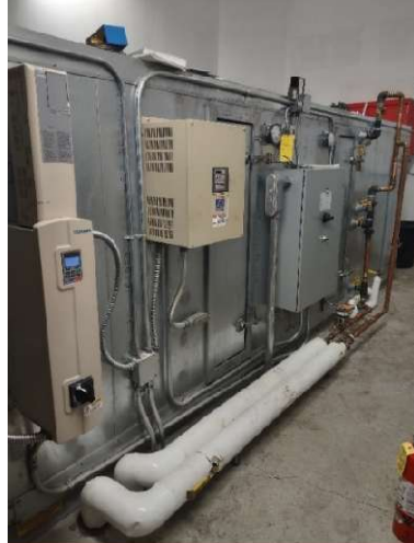
Damper control wiring.
