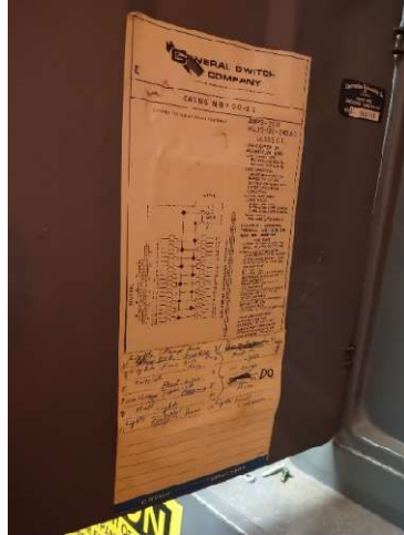
Sub panel original to the facility. Shows signs of age.
