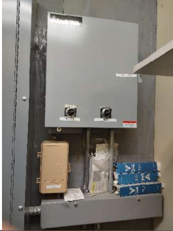
Panel for lighting and outlets – typical.
