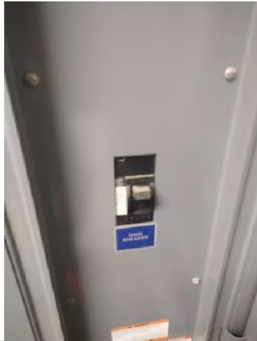
Panelboard shows signs of age.
