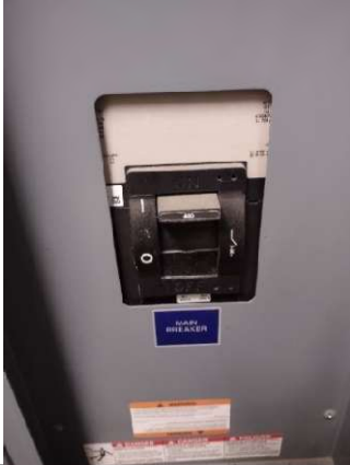
Panelboard for boiler room.
