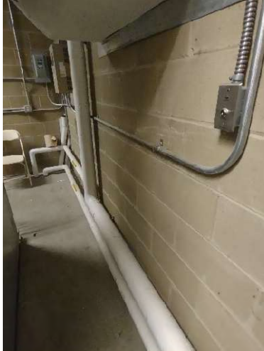
Gym ductwork arrangement and large fans.
