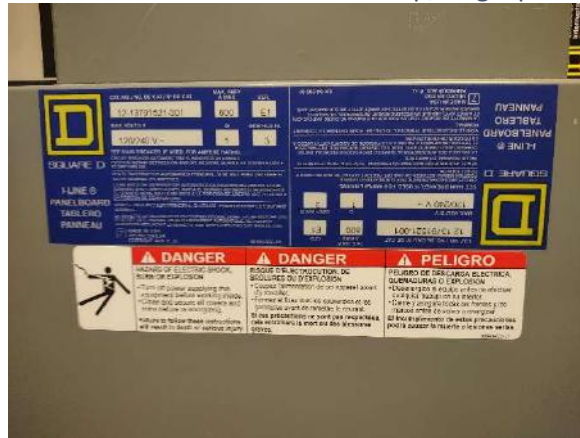
400 amp disconnect-double trouble safety switch for a generator. Switch is off.
