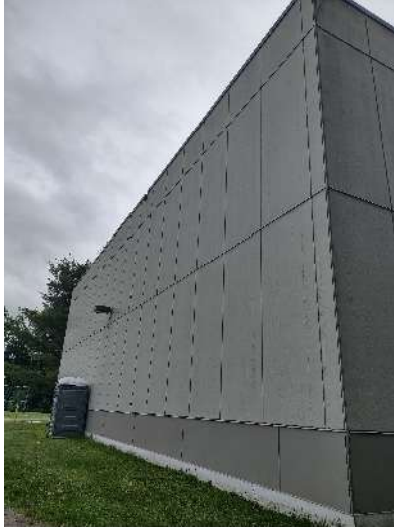
Exterior flood lights to be upgraded.
