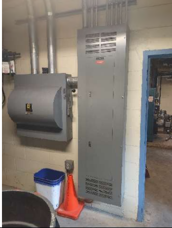
Old main circuit breaker.
