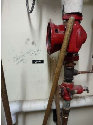
Hot water piping through gym to upper AHU Room.
