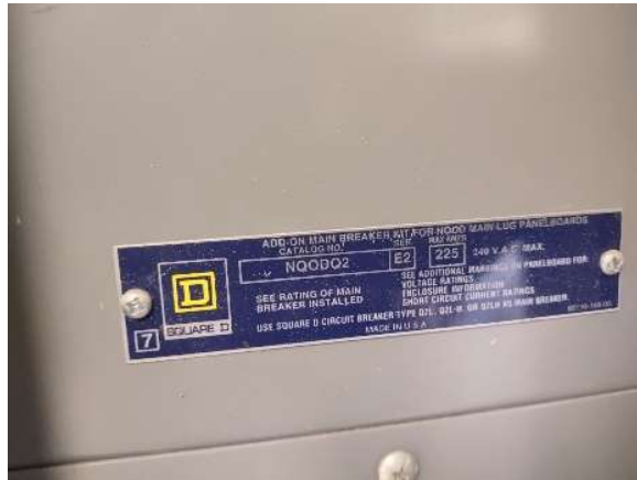
Main breaker showing signs of age.
