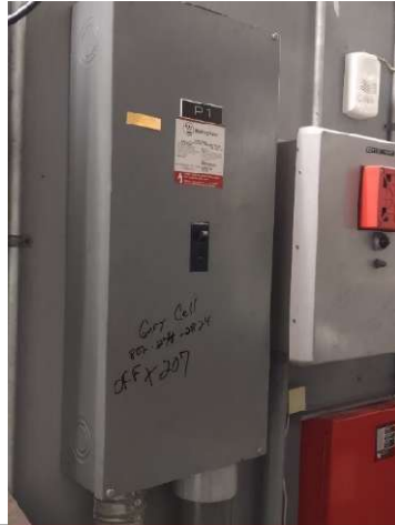
200 amp, 120/240 volt, main breaker – AHU room.
