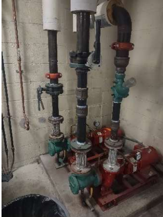
New auto control valves – Very good condition
