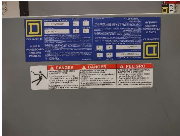
Older panelboard with fire emergency circuit.
