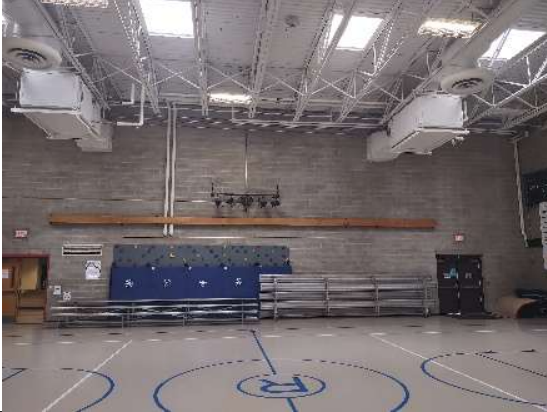
Piping connection to AHU.
