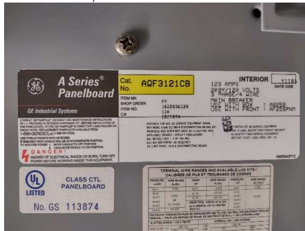
Hallway lighting subpanels - typical.
