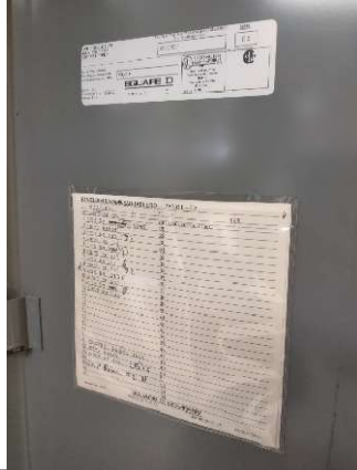
Older main breaker.
