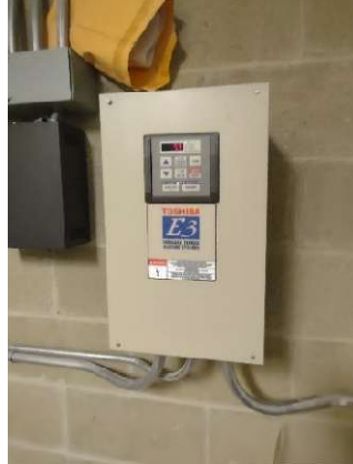
AHU Room above boiler room – auto shut off switch.
