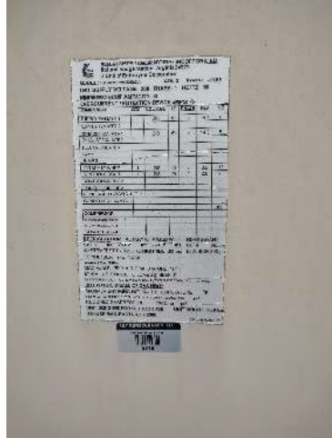
RTU on roof
