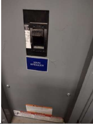
Panelboard for kitchen.
