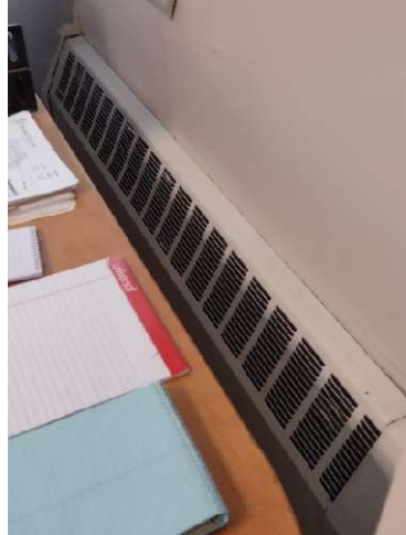
AHU room equipment
