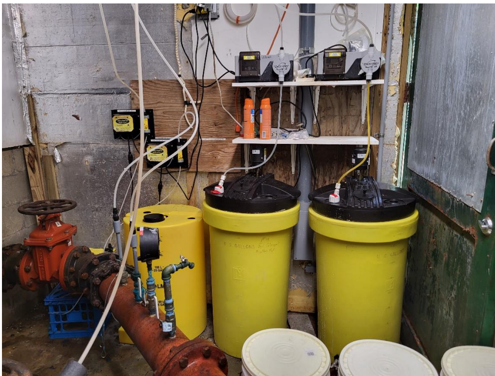
Photo 5 – Existing chemical feed equipment for Wells GPW 1 and GPW 2 in Well GPW 1 pump house. Taken 6/27/23
