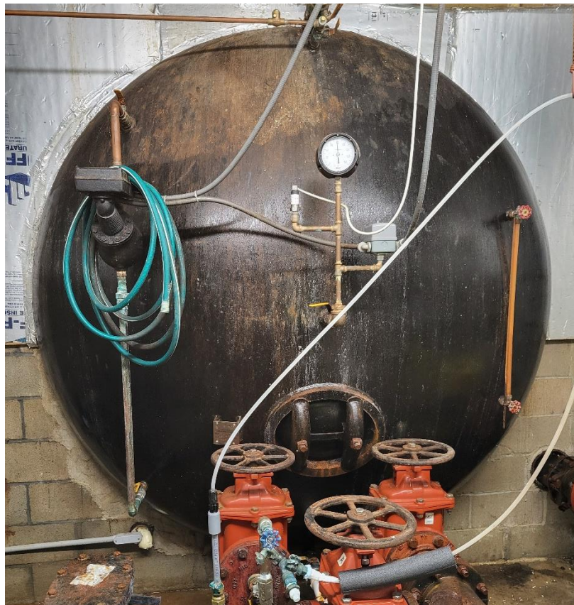
Photo 4 – Existing hydropneumatic storage tank in Well GPW 1 pump house. Taken 6/27/23
